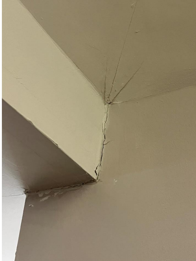
Middleburg Photograph 3 – Interior Cracks
