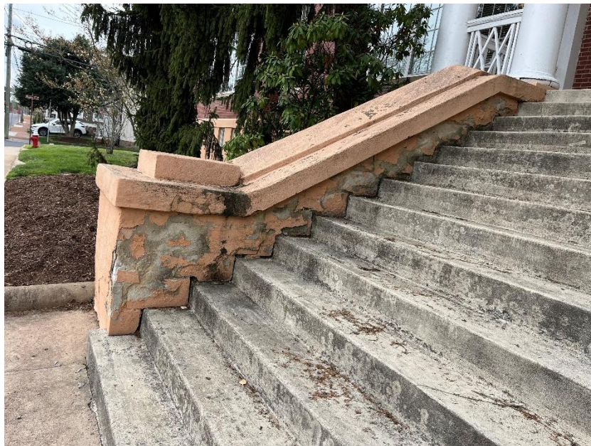
Administration Photograph 2 – Side Rail Separation / Spalling
