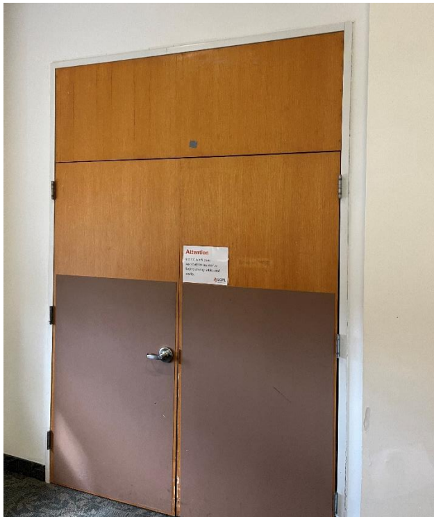
Cascades Photograph 2 – Door with Movement Issues
