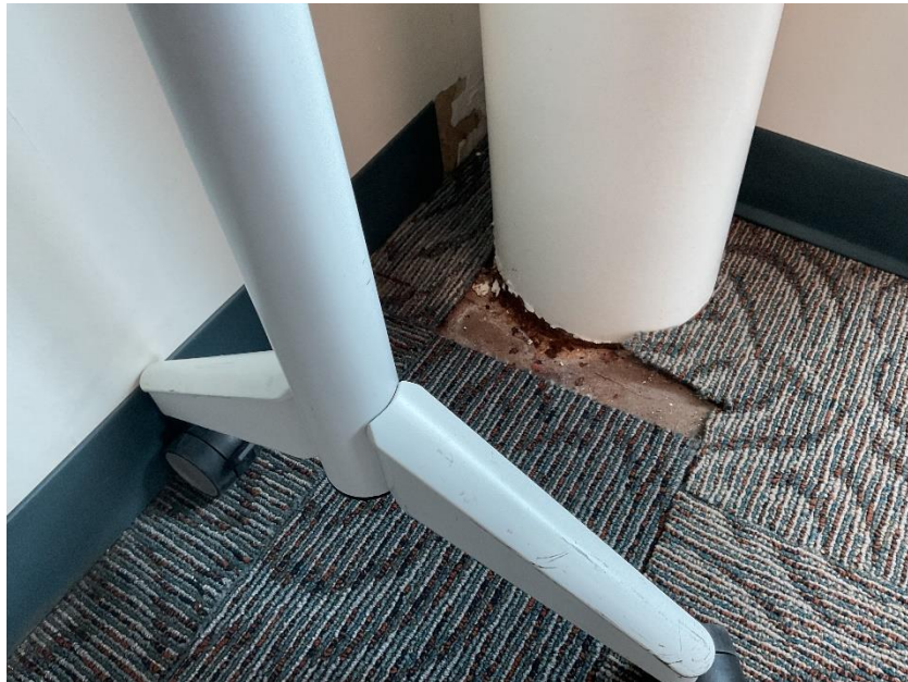
Ashburn Photograph 2 – Interior Column Corrosion at Base
