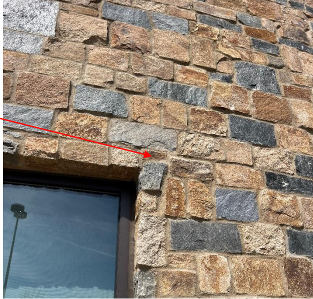
Brambleton Photograph 1 – Diagonal Crack in Stone Veneer
