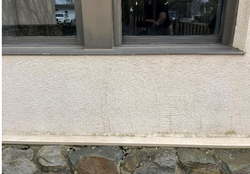
Purcellville Photograph 4 – Stucco Cracks
