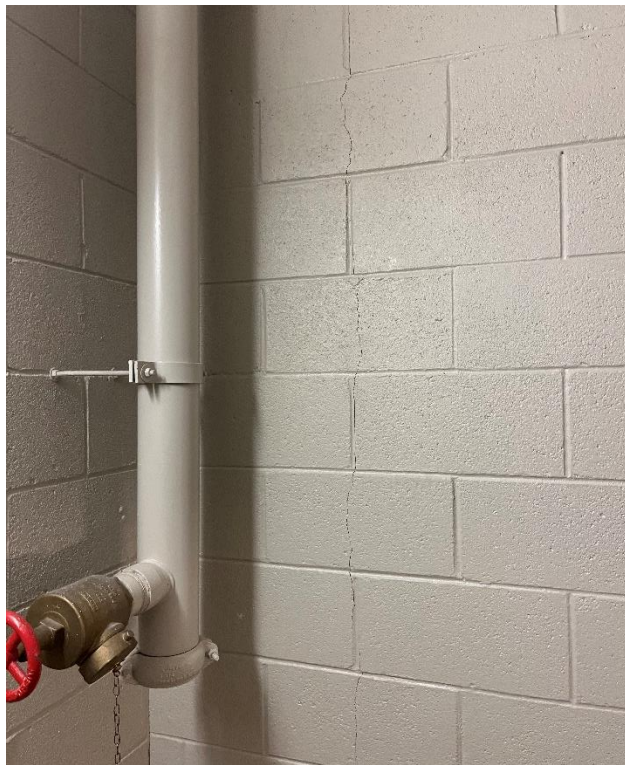
Gum Spring Photograph 2 – Vertical Crack in Stair Shaft
