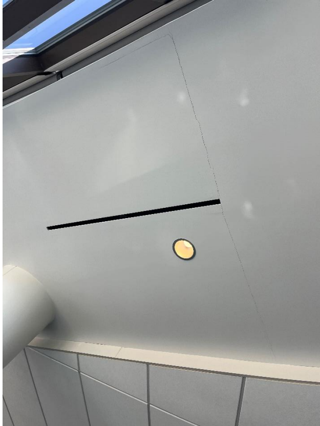
Brambleton Photograph 3 – Crack in Interior Finishes
