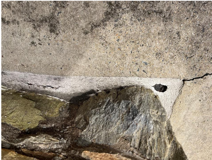
Purcellville Photograph 3 – Damaged Sealant
