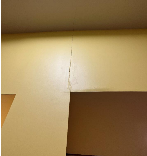
Gum Spring Photograph 1 – Crack in Interior Finishes
