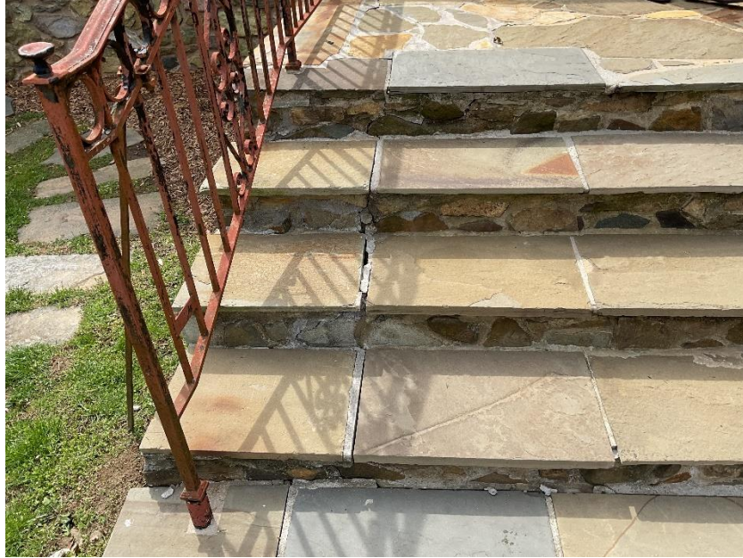
Purcellville Photograph 6 – Damaged Exterior Stair
