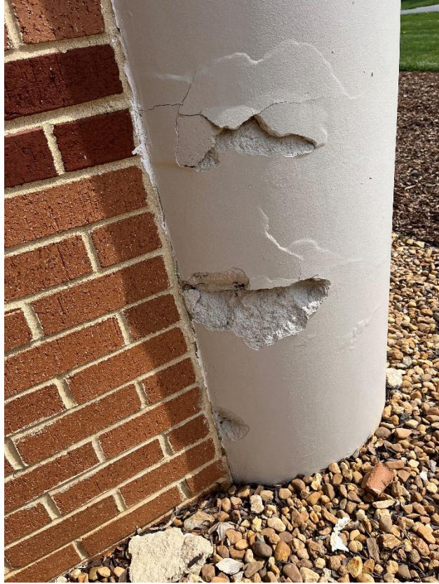
Rust Photograph 1 – Damaged Concrete at Column
