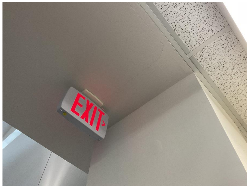
Purcellville Photograph 5 – Cracks in Interior Finishes
