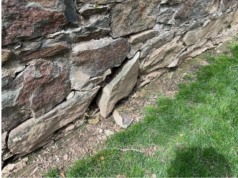
Purcellville Photograph 2 – Loose Stones in Wall
