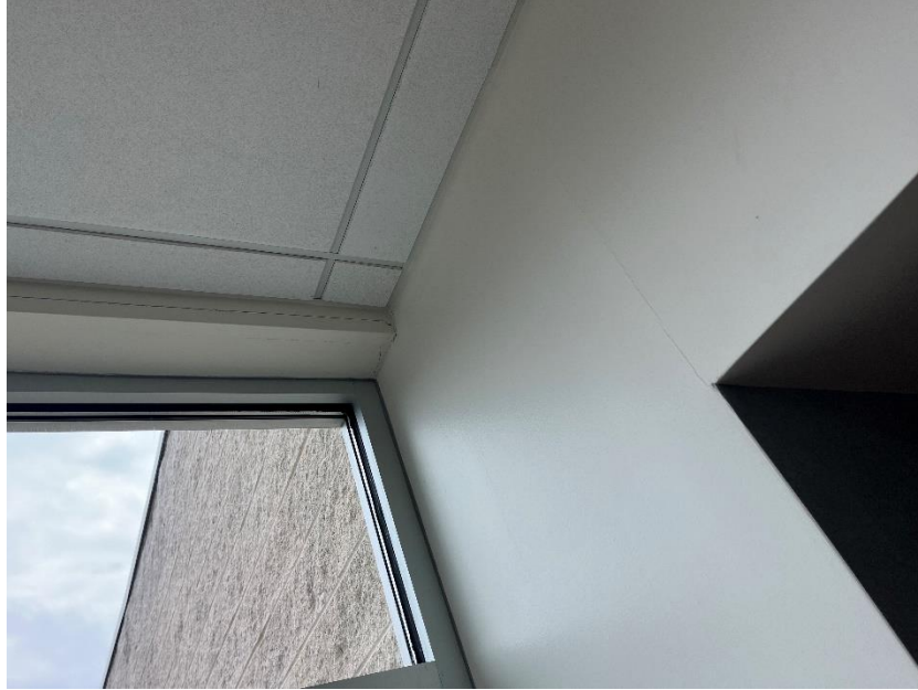
Ashburn Photograph 5 – Crack in Interior Finishes
