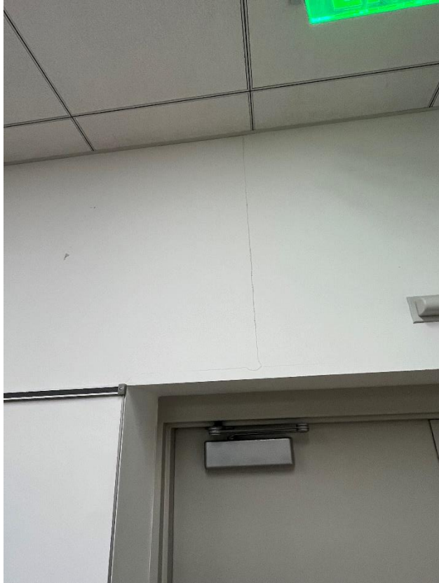
Sterling Photograph 3 – Crack in Interior Finishes
