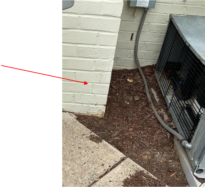
Lovettsville Photograph 1 – Diagonal Crack in Brick Veneer
