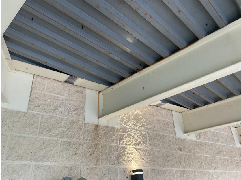
Ashburn Photograph 1 – Exterior Steel Corrosion
