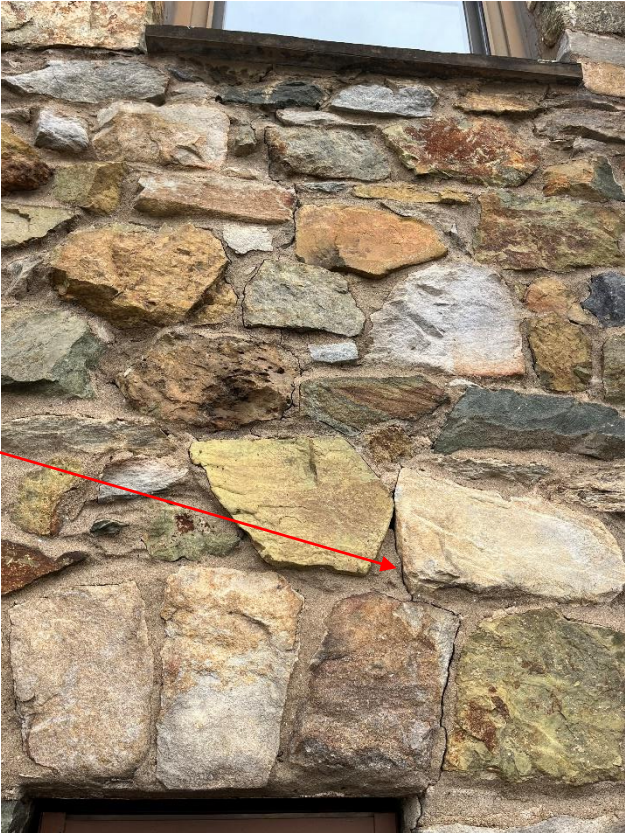
Purcellville Photograph 1 – Crack in Stone Wall
