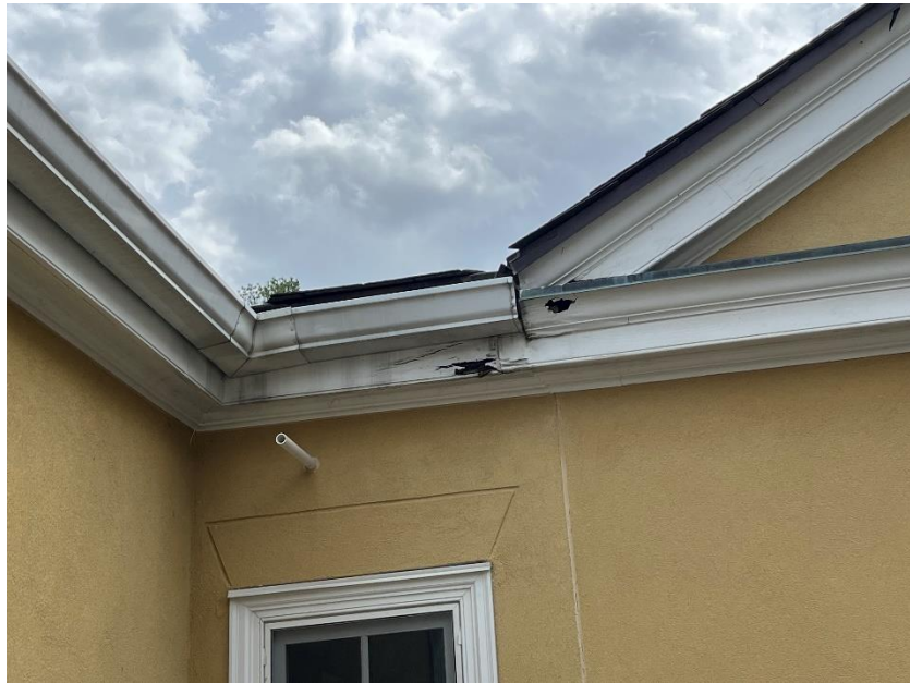
Middleburg Photograph 2 – Fascia Board Rot (North Side)
