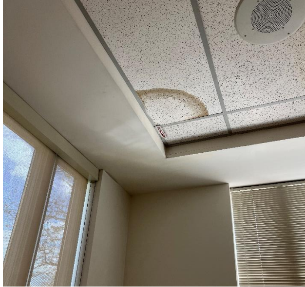
Cascades Photograph 5 – Moisture Damage at Ceiling Tiles
